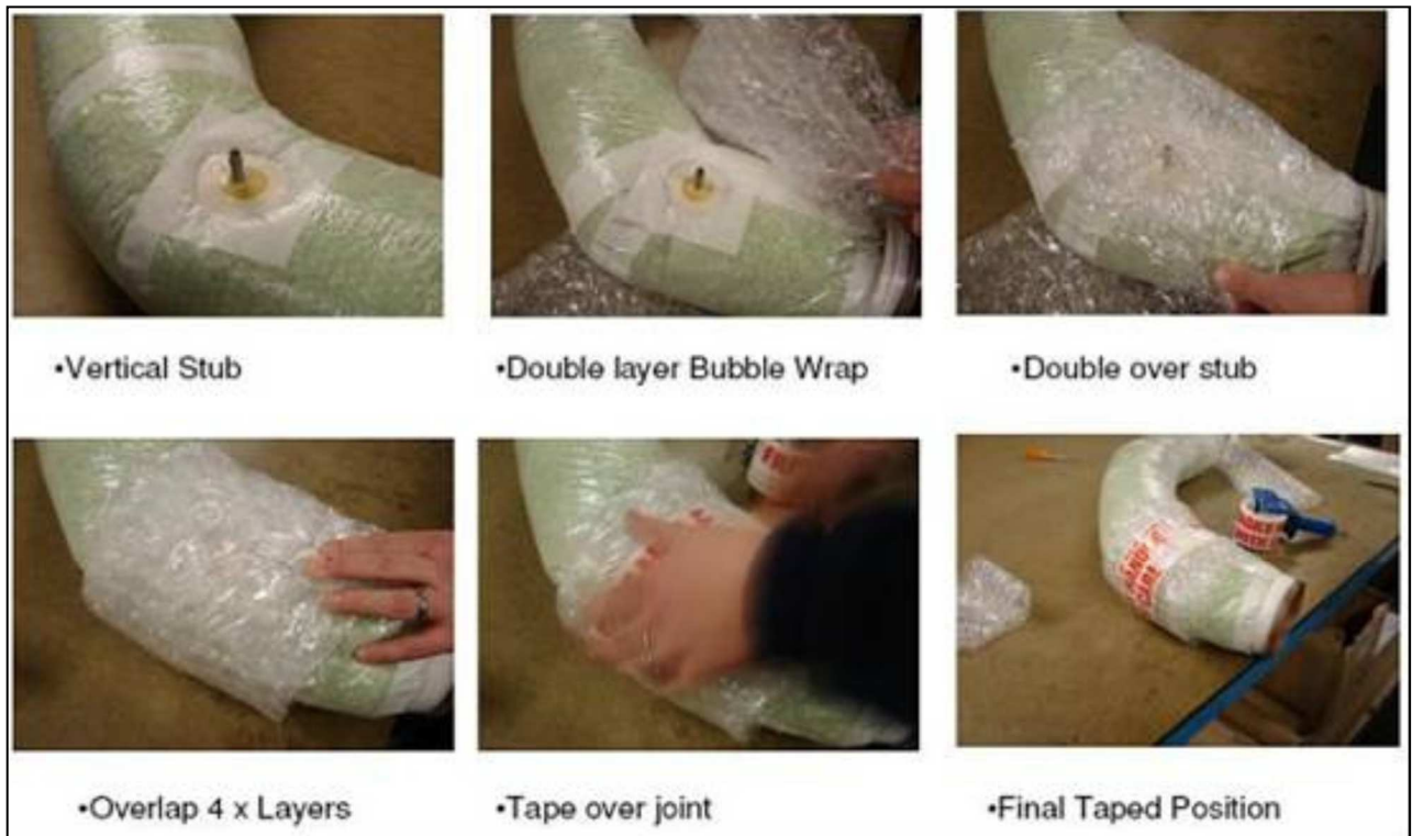
Figure 73: Example of sharp point protected
